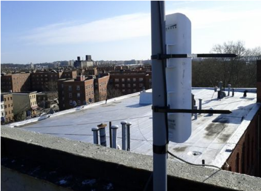
Figure CsOTI 6: Node installed on the roof of an apartment building.
