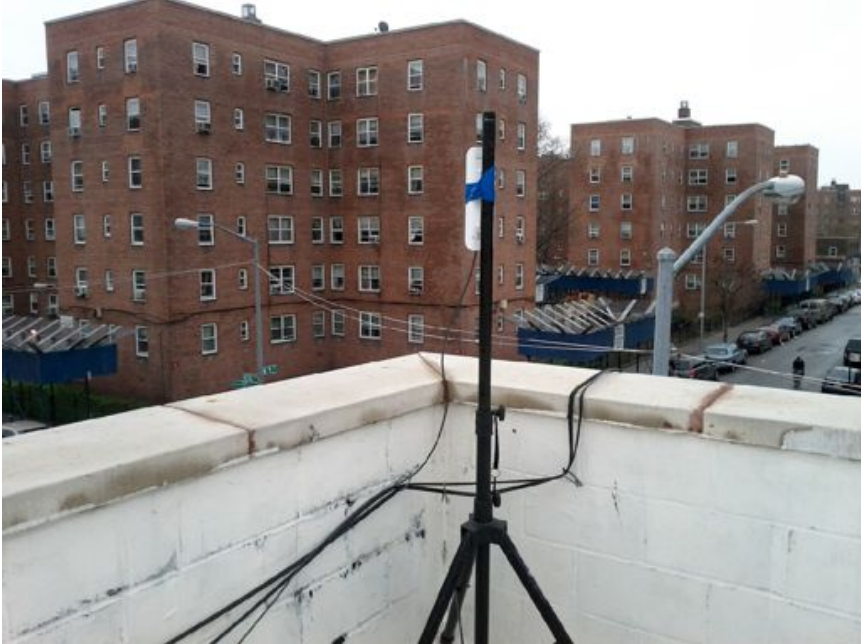
Figure CsOTI 4: First RHI WiFi node (Ubiquiti Nanostation) installed on the rooftop of the building that houses the RHI offices.
