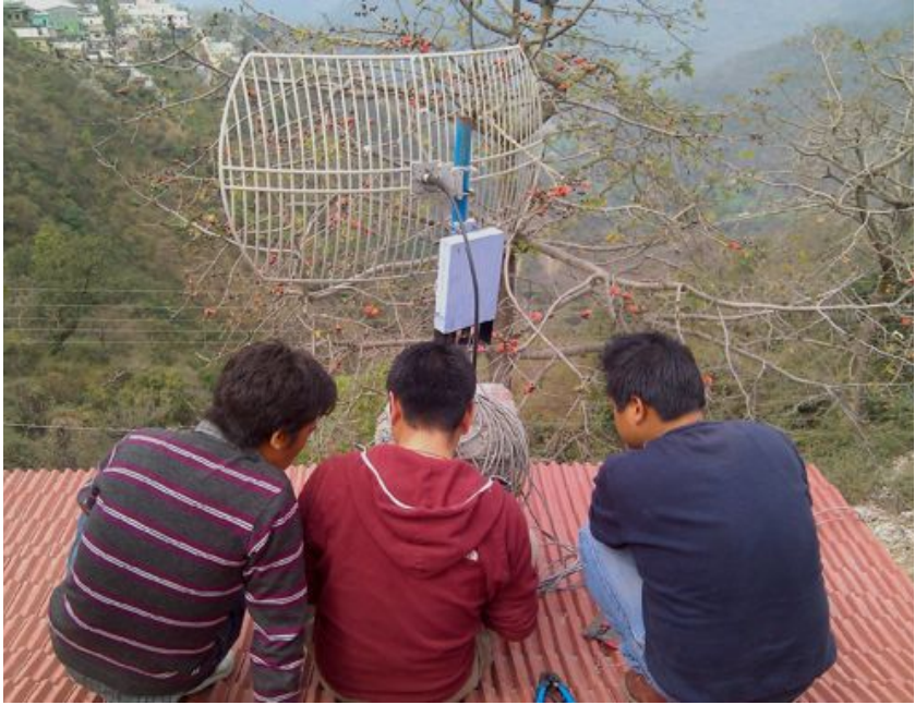
Figure CSD 6: Relay troubleshooting, Kumaon Network
