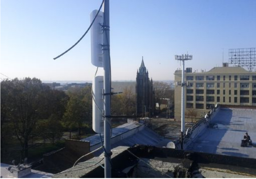
Figure CsOTI 14: Rooftop node installed after Superstorm Sandy.
