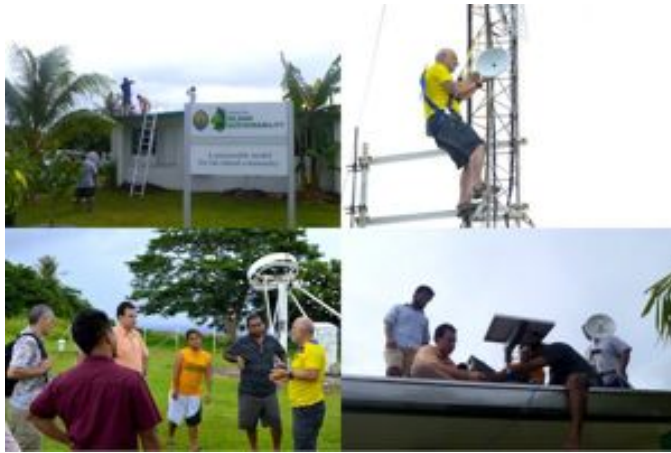
Fig. CSP 2: A new faster Internet connection for the Centre for Island Sustainability
