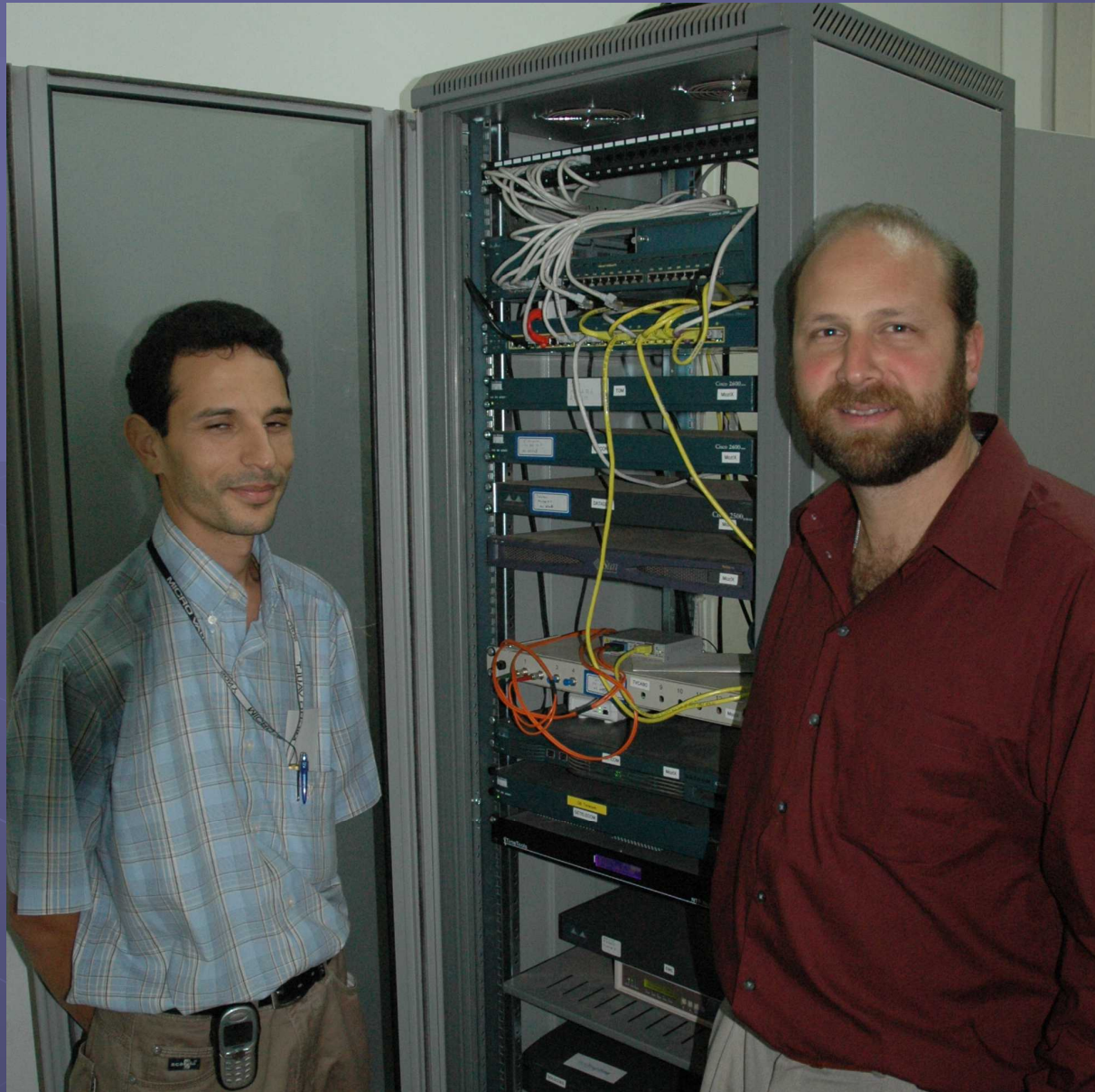
Mozambique Internet Exchange, Maputo
